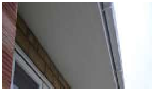
Pieces of Asbestos Insulating Board (AIB)
