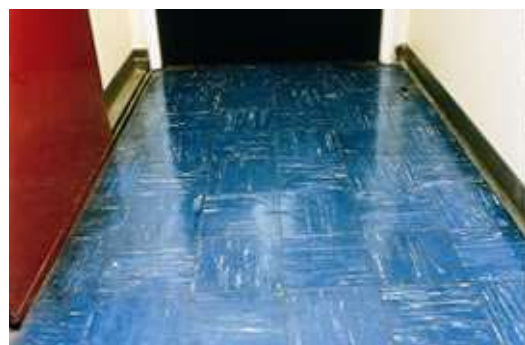
Asbestos containing floor tiles in a corridor
