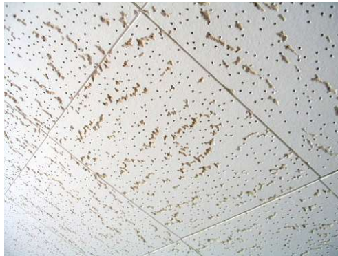
Asbestos containing ceiling tiles
