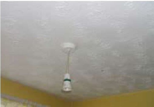
Asbestos textured coating
